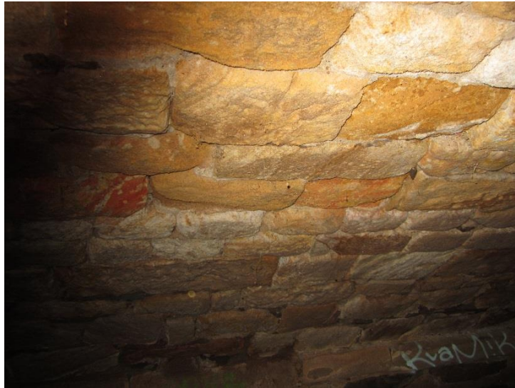
Figure 13 - Degradation of the mortar between the sandstone blocks
