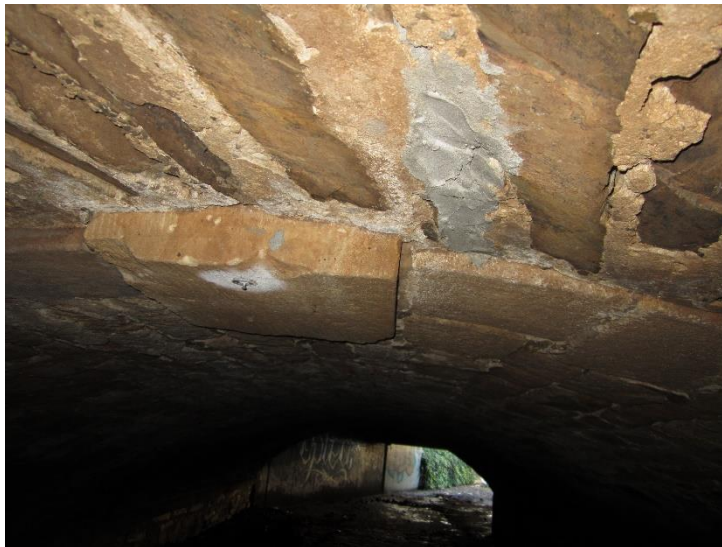
Figure 14 - Previous attempts to repair structure
