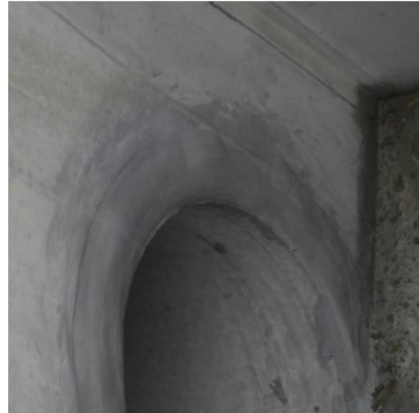
Figure 19 inside connection of the pipe with the pit using site-approved cement mix
