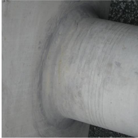
Figure 18 Outside connection of the pipe with the pit using site-approved cement mix(Humes 2012)
