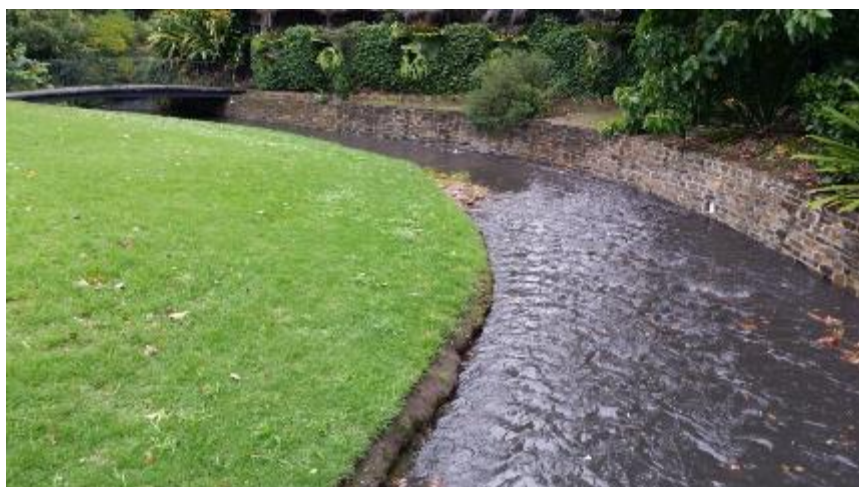
Figure 76: Eroded Creek bank (submerged) and concrete retaining wall (right of picture) typical of Section 3 (Hydro-Future 2015)
