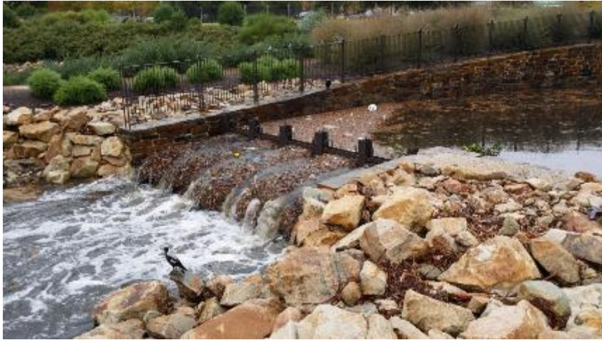
Figure 84: Channel or Creek Net used in the transition from Section 5 to Section 4. (Hydro-Future 2015)
