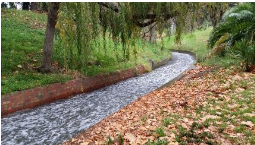
Figure 74: Rectangular Concrete Lined Channel, photo taken after the rain shower (note the rapid water flow) (Hydro-Future 2015)
