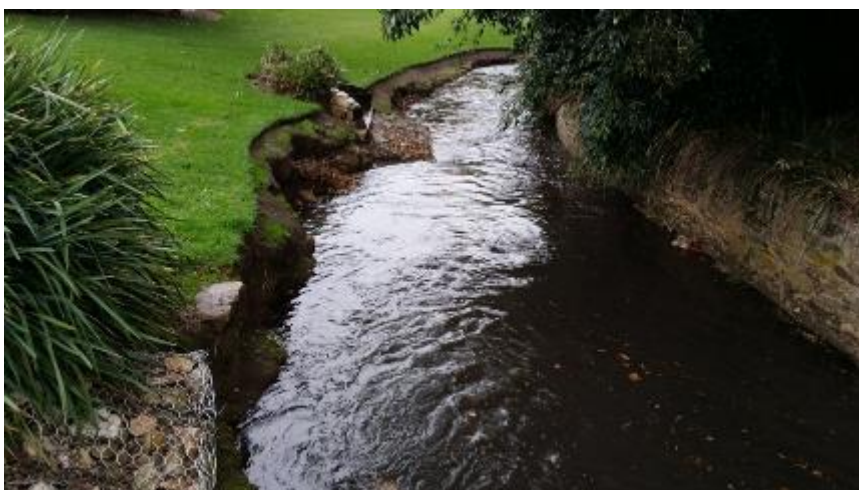
Figure 79: Eroded Creek bank, concrete retaining wall (right of picture) typical of Section 3. Note the two gabion baskets (Hydro-Future 2015)
