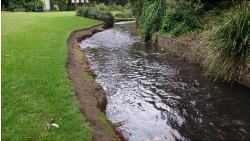
Figure 77: Eroded Creek bank (partially submerged) and concrete retaining wall (right of picture) typical of Section 3 (Hydro-Future 2015). Note steel meshing used to reinforce the soil against erosion (Hydro-Future 2015)
