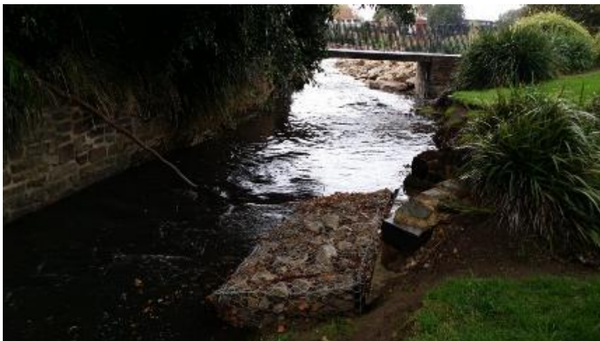
Figure 78: Start of Section 3, note the failed gabion basket in the picture's foreground (Hydro-Future 2015)
