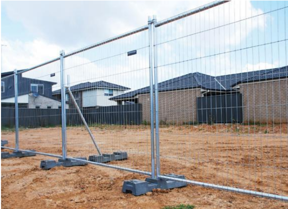
Figure 226 Temporary security fencing around construction site, similar to what will be used around the site yard and site office (CHC 2015)
