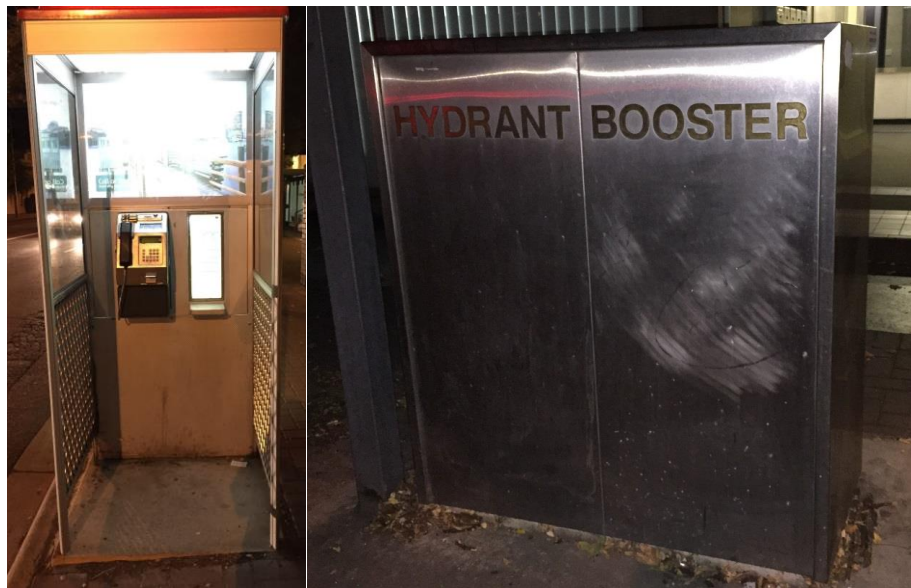
Figure 30: (left to right) Telephone booth and Fire hydrant booster
