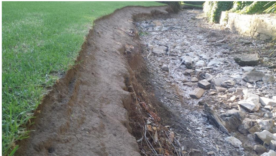
Figure 116: Eroded Creek Bed (Hydro-Future 2015)
