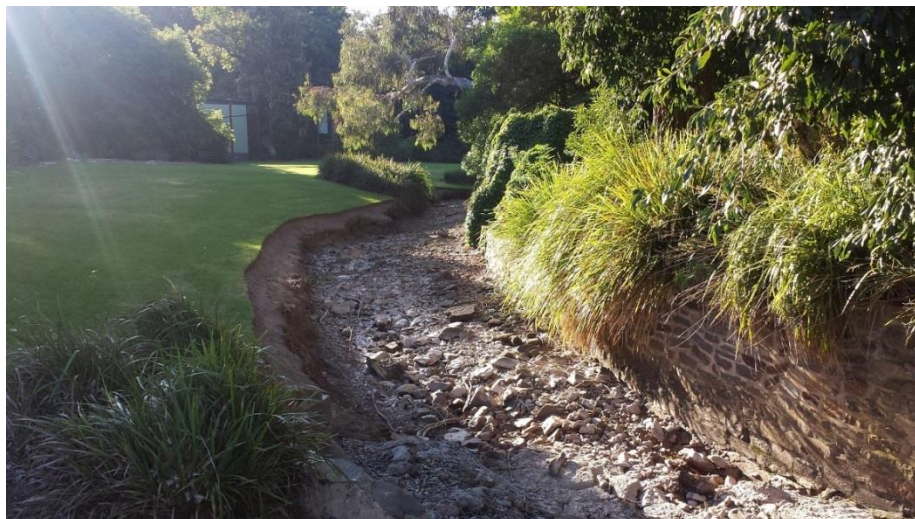
Figure 117: Eroded Creek Bed (Hydro Future 2015)
